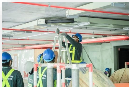
Mechanical and Electrical
